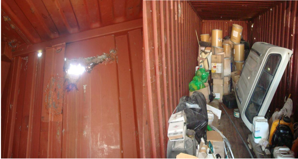
Figure 2. Degraded conditions of storage shed at Corozal Vector Control
