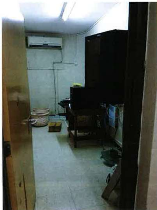
Figure 60: Server room - proposed room for PV equipment at Winston Scott Polyclinic
