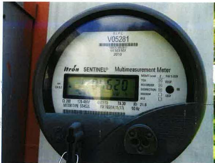
Figure 32: Electricity utility meter at the Edgar Cochrane Polyclinic
