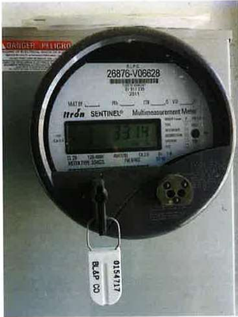
Figure 46: Utility meter at the St. John Polyclinic equipment
