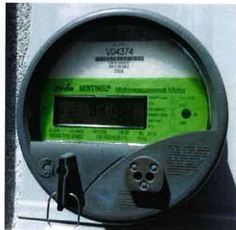
Figure 54: Utility meter at St. Philip Polyclinic
