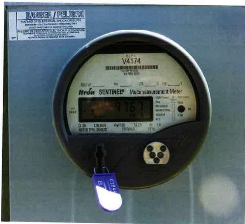
Figure 18: Electricity utility meter at Maurice Byer Polyclinic
