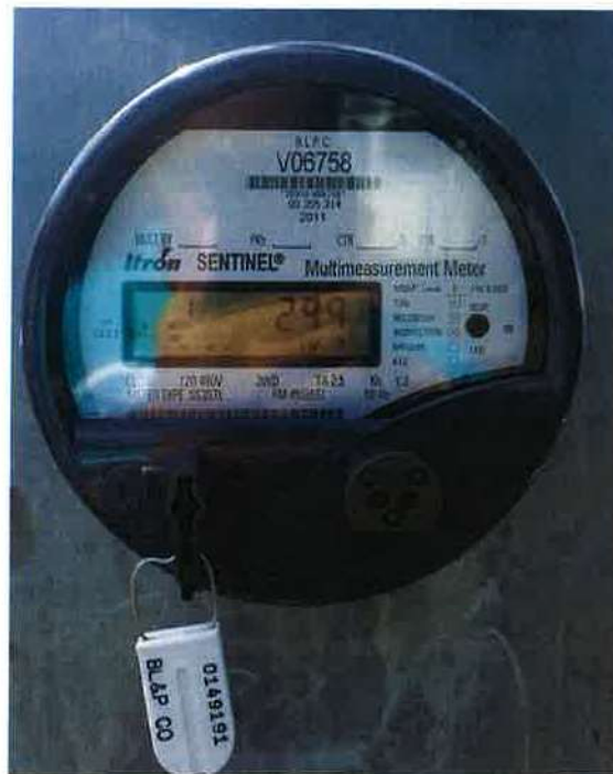
Figure 39: BLPC Utility Meter at Brandford Taitt Polyclinic
