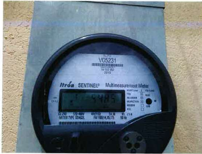
Figure 6: Utility Meter at Eunice Gibson Polyclinic
