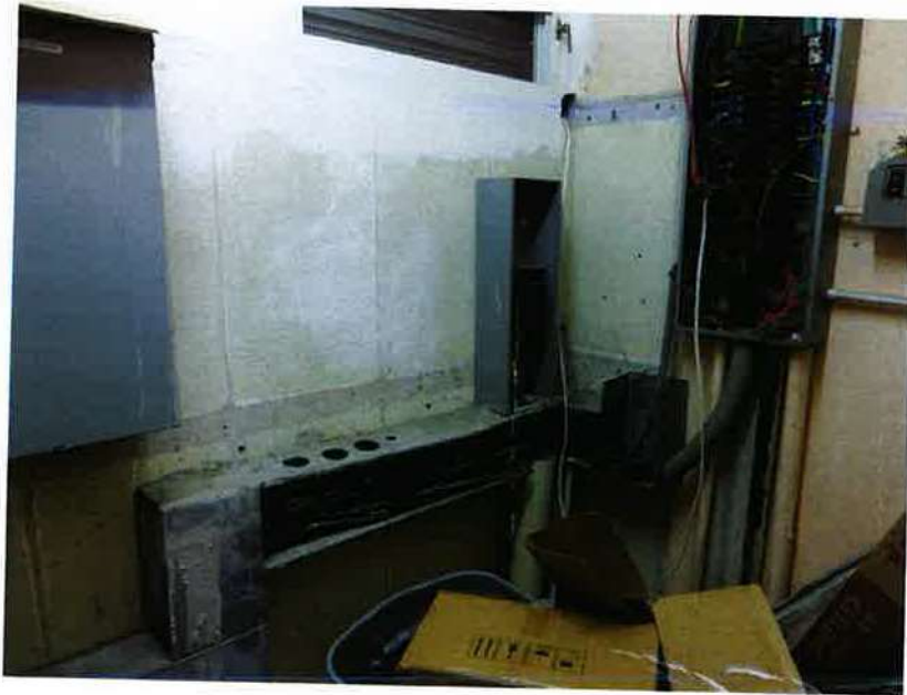
Figure 17: Main electrical panel room - proposed location for PV equipment
