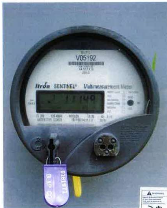
Figure 25: Electricity utility meter at the Glebe Polyclinic
