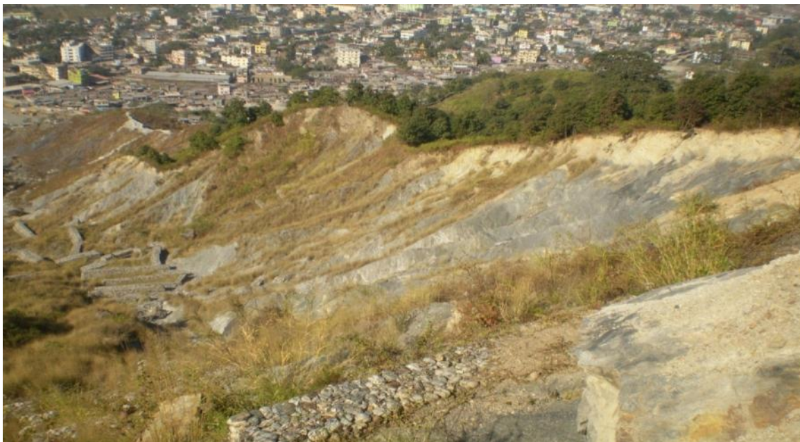
Figure 6, Photograph showing the different stages of landslide in the NW of Rinchending Goenpa area over residential areas
