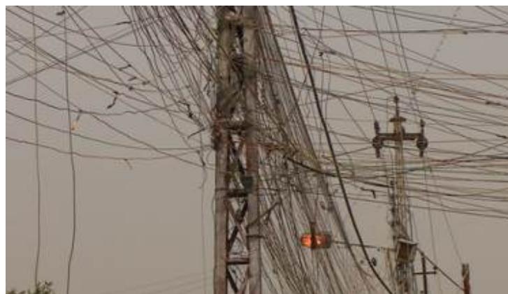
Figure 2. Ad-hoc power distribution grids established by entrepreneurs who run diesel generators to feed demand when the grid is down.
