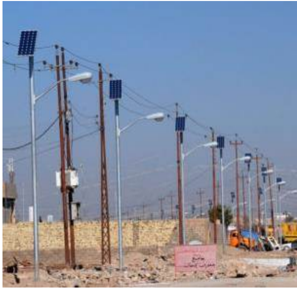
Figure 9. Solar street lights installed in Baghdad.
