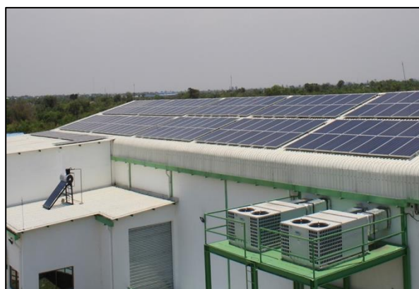
Fig. 3: Medical Warehouse Zâmbia, with Solar system installed. In Zâmbia, UNDP installed Solar Systems at all four Regional Hubs.
