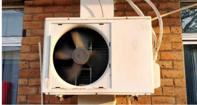
Figure 35 Air conditioner installed in a Central Healthcare facility
