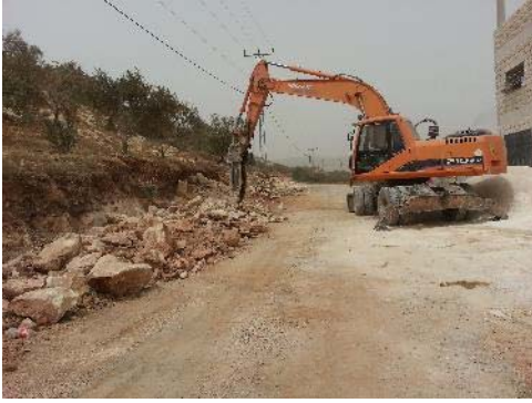
Aqraba Connecting Road
