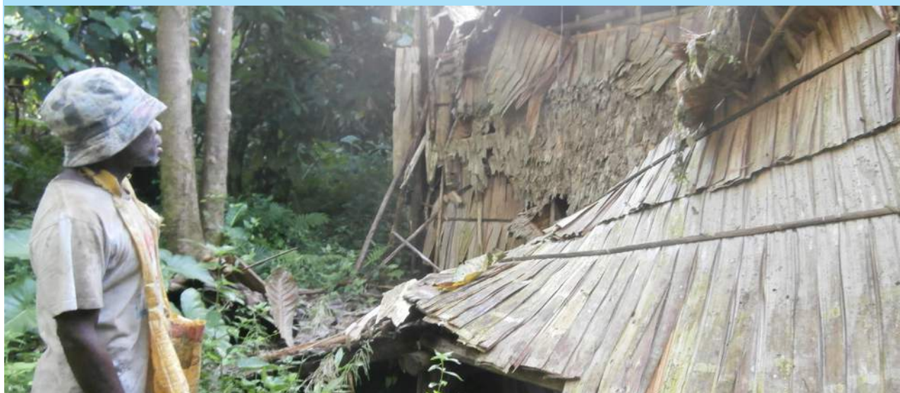
UNDP/Adi Galokepoto/ Damaged house in Marunga village.
