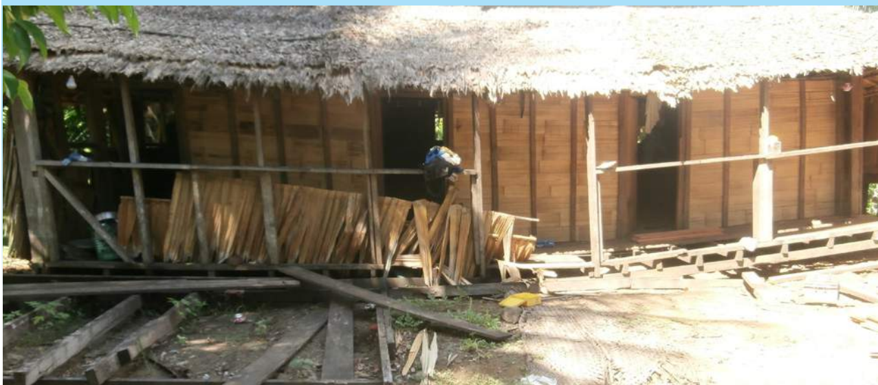
UNDP/ Adi Galokepoto/ Partly damaged house at Parego village.
