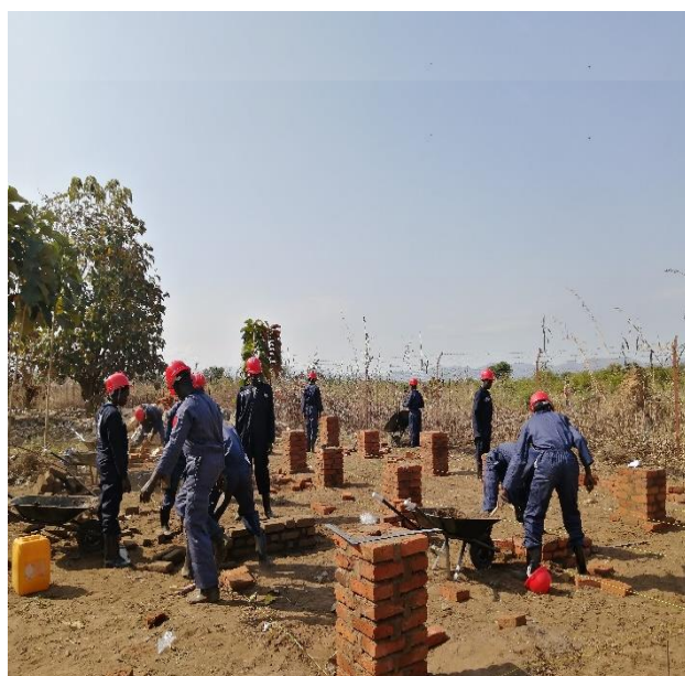
Students taking part in Masonry and brick laying training at Torit VTC (December 2019, UNDP)
