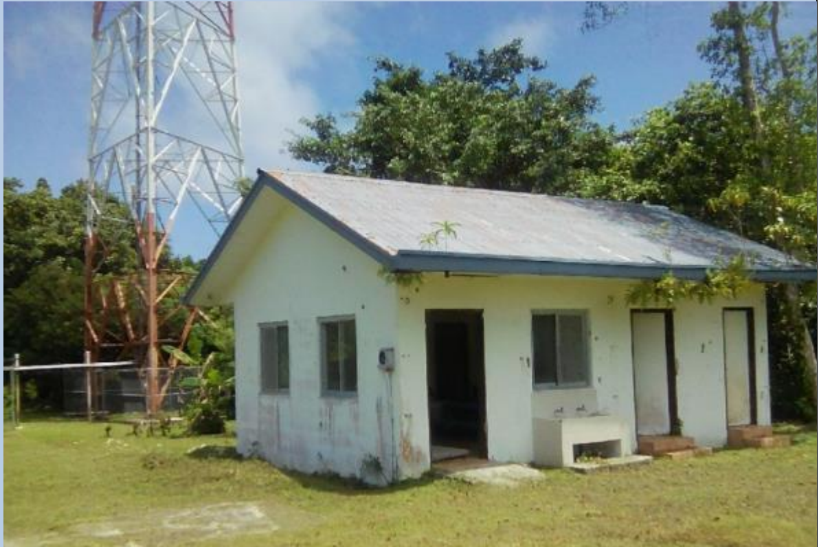
Figure 35 Photo (UNOPS) showing the proposed site building for refurbishment into small health centre. Due to the small population size, a small health centre is appropriate, and easier to manage and maintain.
