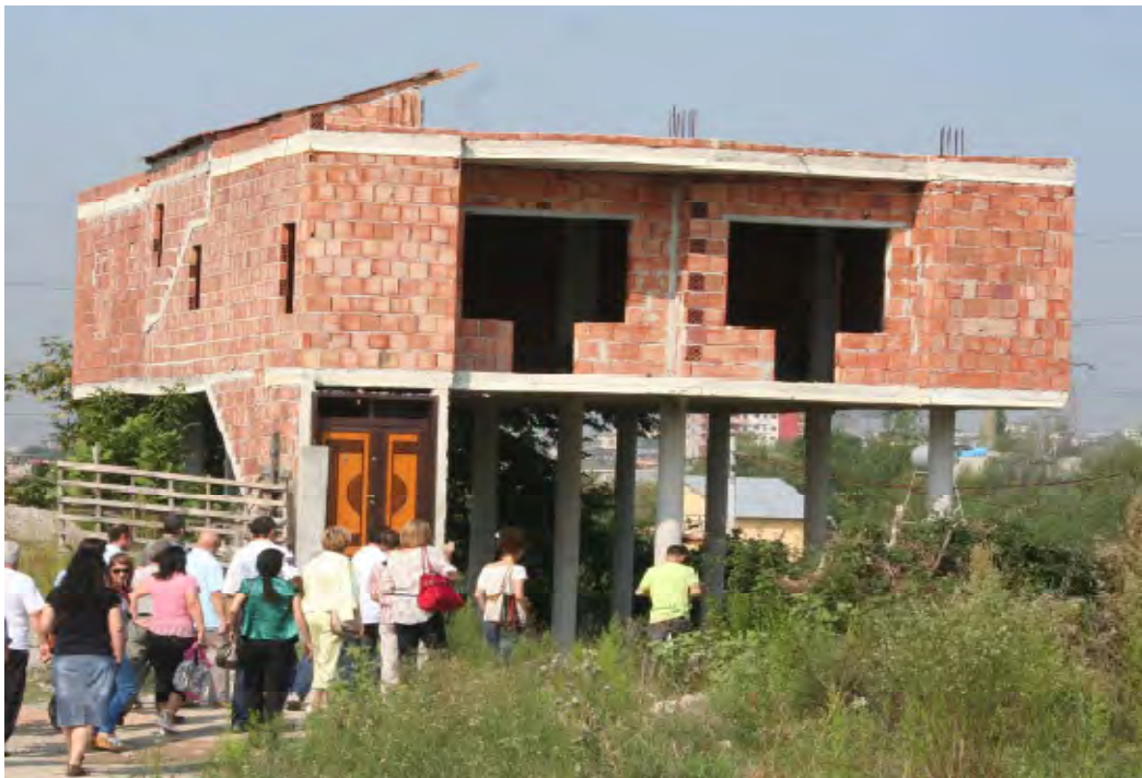
Photo 8: New unpermitted house being constructed on fill in Tirana River floodplain
