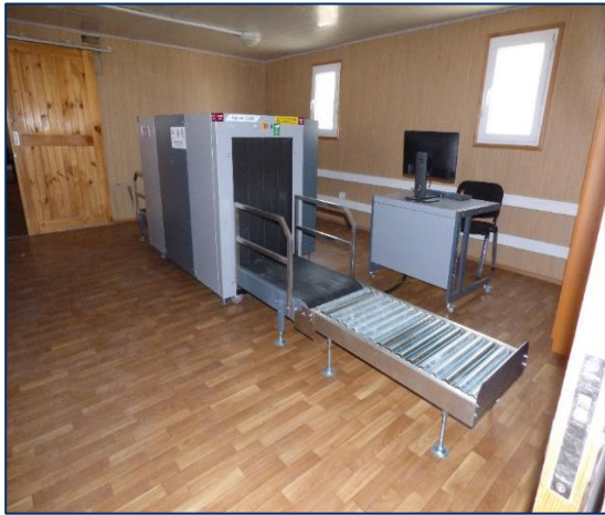
X-Ray scanner installed at BCP
